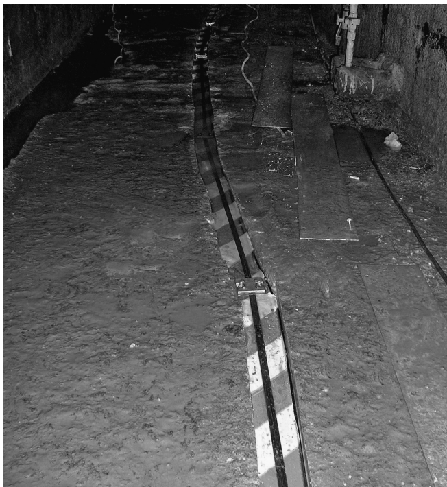
Figure 6. Strain sensor installation in the Plavinu Dam inspection gallery.
