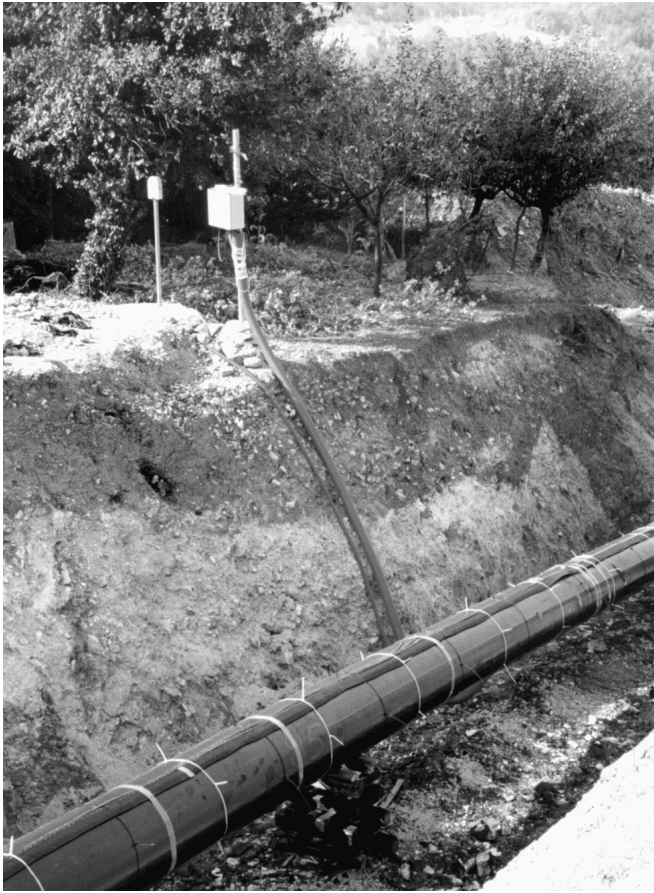
Figure 7. Strain and temperature sensing cables installed on a gas pipeline. The picture shows a sensor line attached to the top of the pipeline and one on the side. The sensors are protected with an black neoprene pad. Another sensor line is attached symmetrically on the opposite side. The temperature sensing cable is also installed on top of the pipe. The vertical tube at the center of the picture, brings the optical cables from the pipeline to the junction box.
